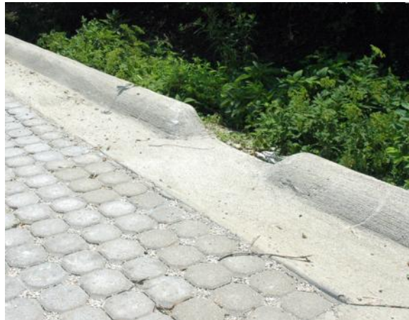
Figure 12-B: Cuts in the continuous curb allow for stormwater to be directed into landscaped areas.
